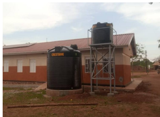
Rain water harvest with solar pump.
